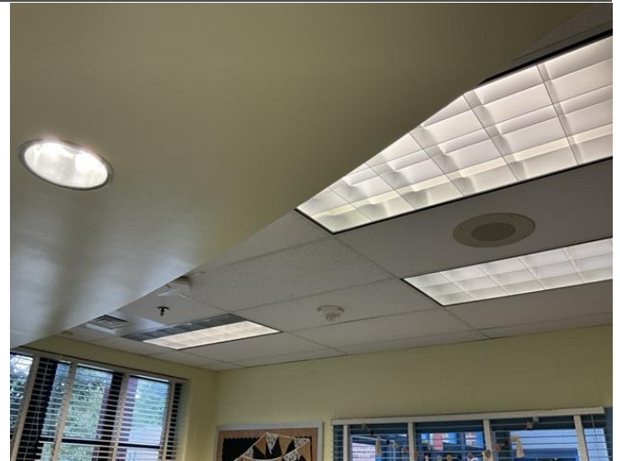
26 - INTERIOR LIGHTING SYSTEM
