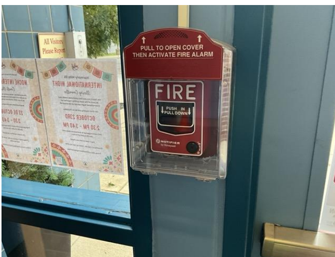
29 - FIRE ALARM SYSTEM
