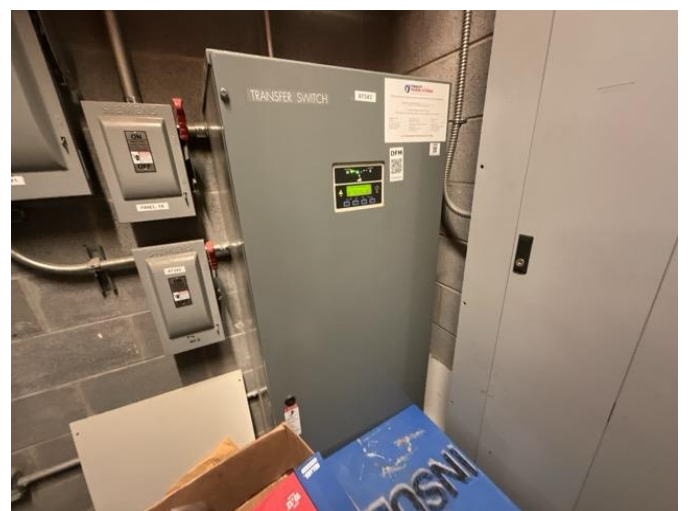
24 - AUTOMATIC TRANSFER SWITCH
