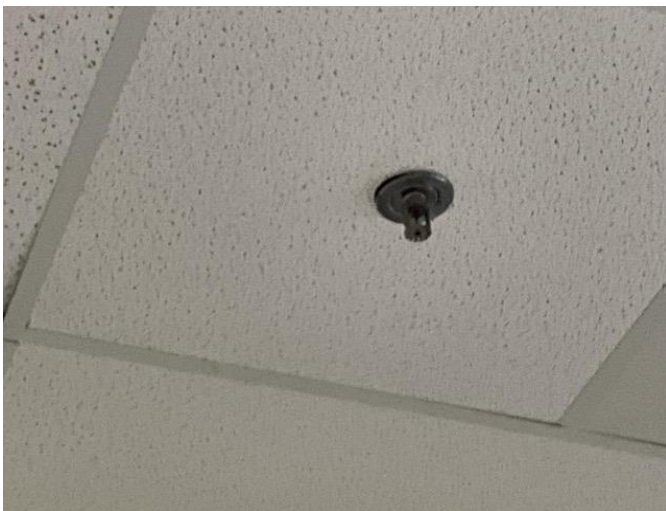
27 - FIRE SUPPRESSION SYSTEM
