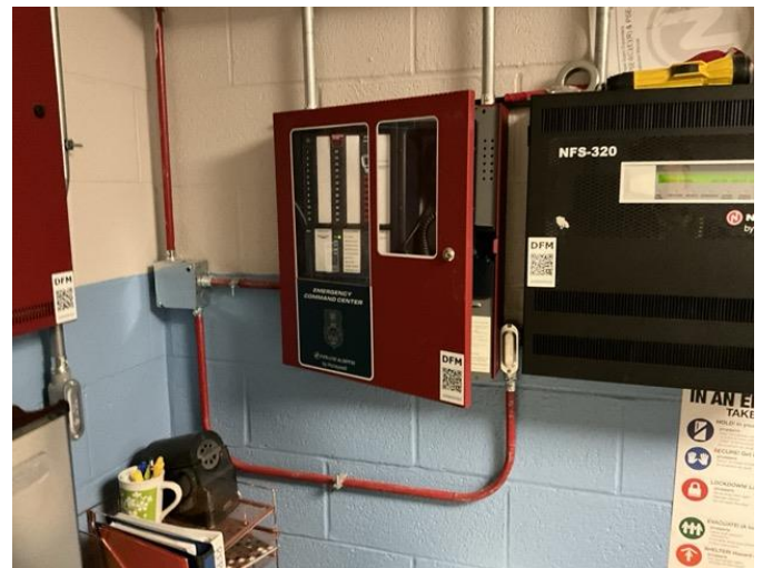
28 - FIRE ALARM PANEL
