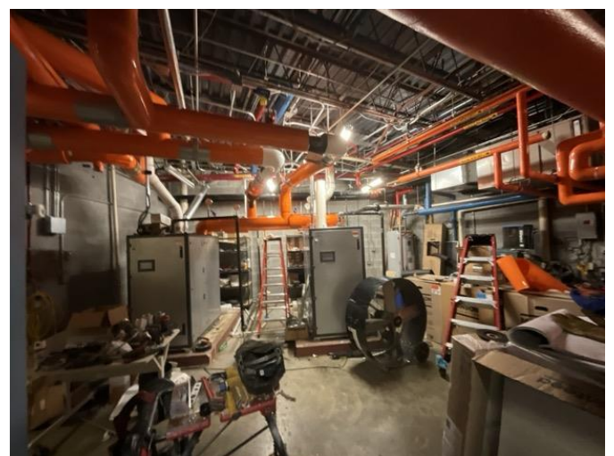
18 - MECHANICAL ROOM, BOILERS
