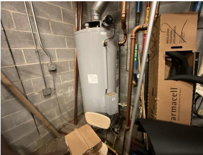
21 - HOT WATER HEATER
