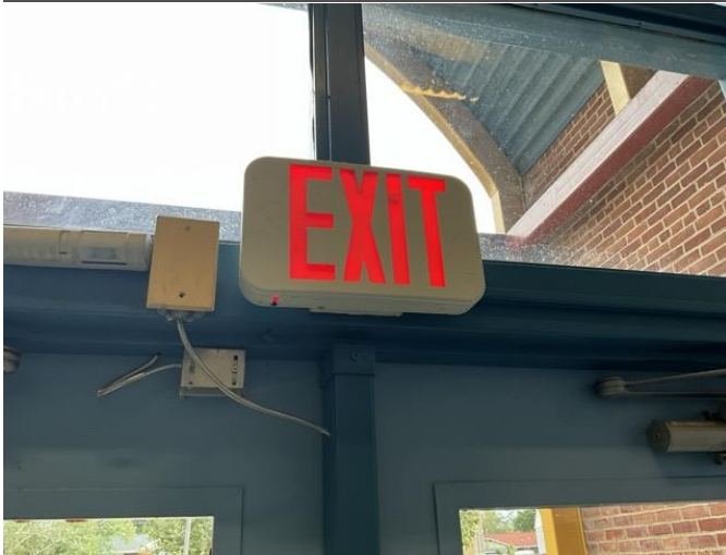
25 - EMERGENCY AND EXIT LIGHTING SYSTEM
